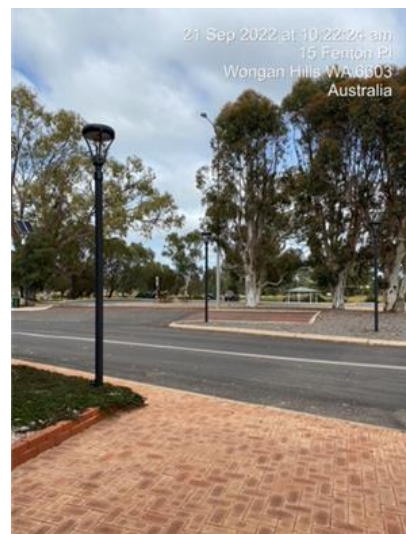
Solar Street Lighting – Fenton Place
